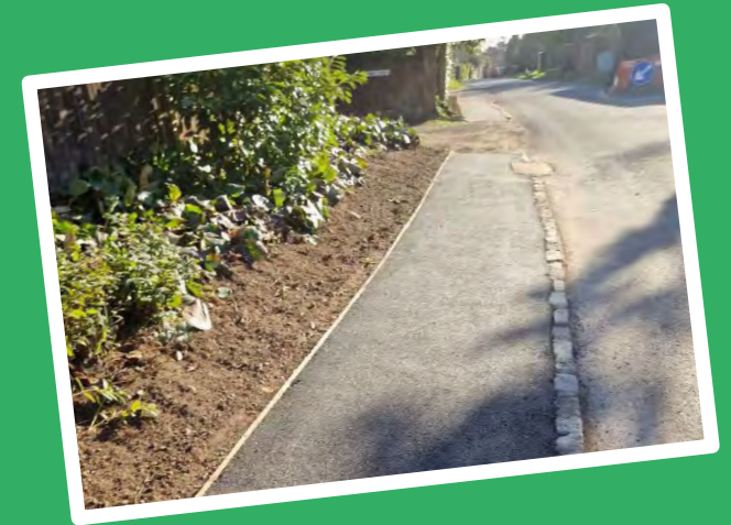
Footway on Blackpond Lane
